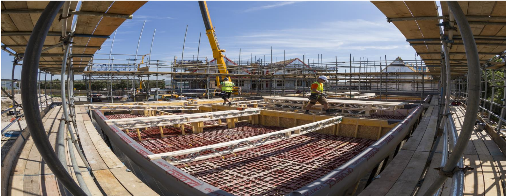
Military Road New Build: This will provide 28 homes for affordable rent and 7 homes for shared ownership purchase due for completion between February and June 2018.
